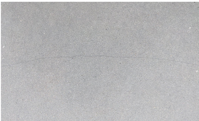
Hairline crack in an Acid Wash finish
